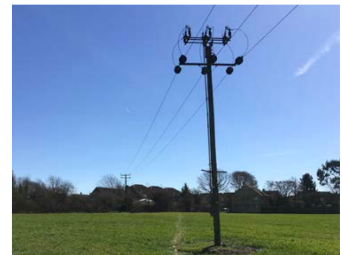
Overhead power lines
